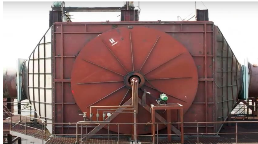
India's first RPC implemented for 75TPH Boiler at Udagiri Sugar and Power Ltd.
